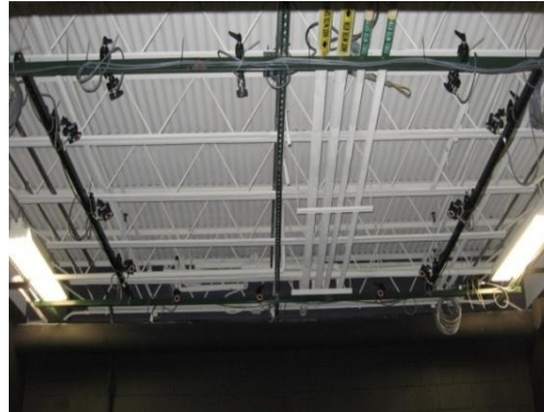
Motion Capture Cameras Attached to the ceiling
